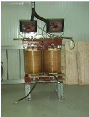
Short-circuit test up to 42kA/2Sec
